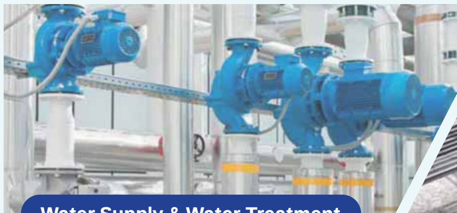
Water Supply & Water Treatment
