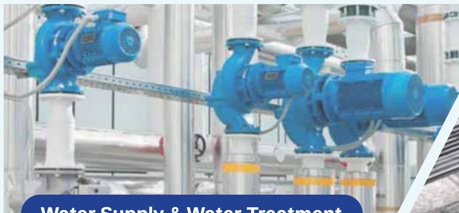
Water Supply & Water Treatment
